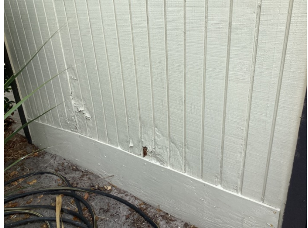
Wood rot at pool house
