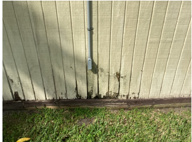
Wood rot at pool house
