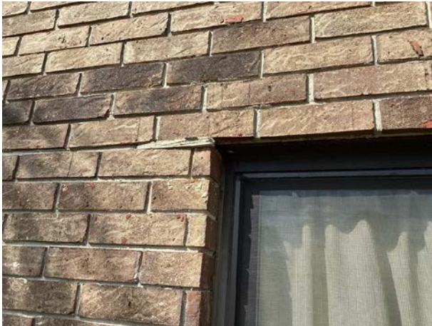
Mortar deterioration at lintel
