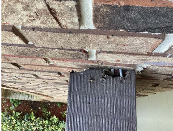
Wood rot at balcony railing
