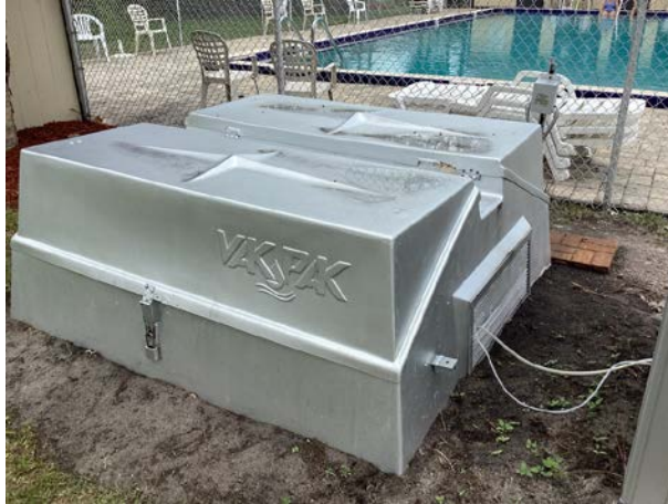
Pool mechanical equipment enclosure
