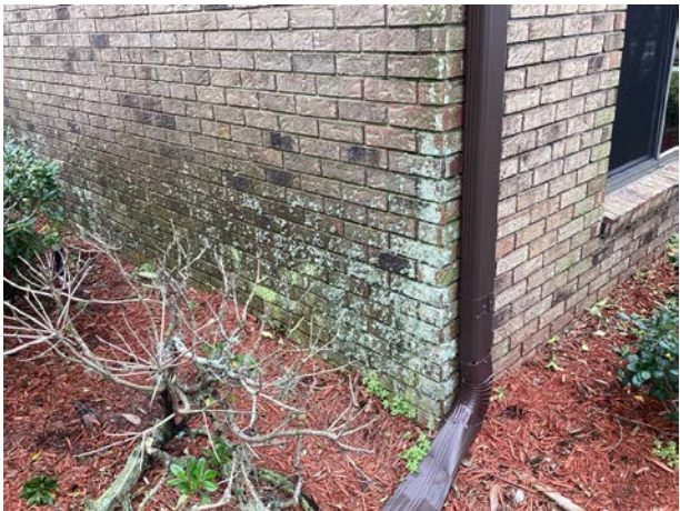
Biological growth at masonry wall
