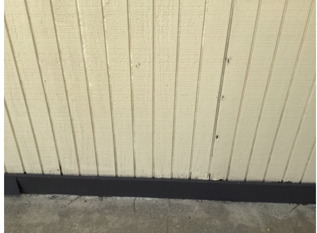
Wood rot at pool house
