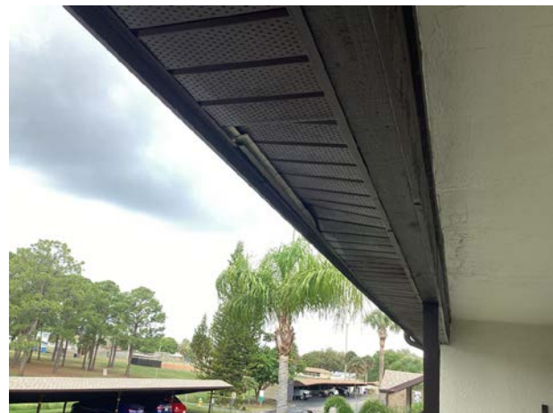
Aluminum soffits and fascia damage
