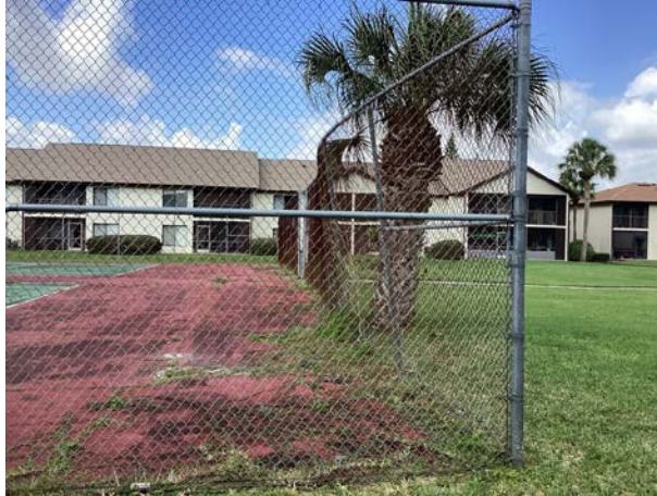
Chain link fence lean
