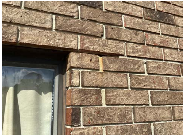
Missing mortar due to rust at lintel
