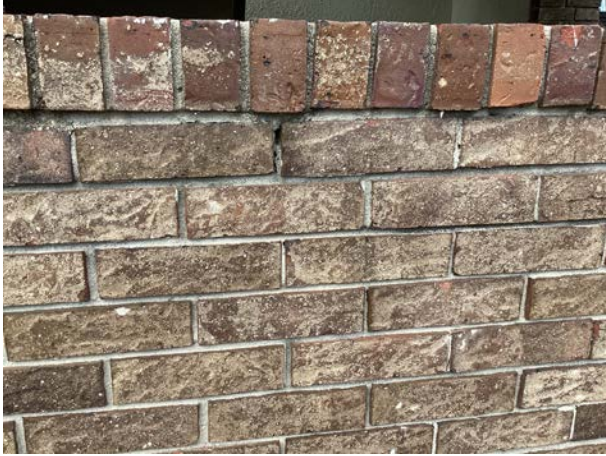
Isolated mortar deterioration
