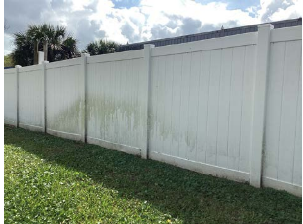
Biological growth at vinyl fence
