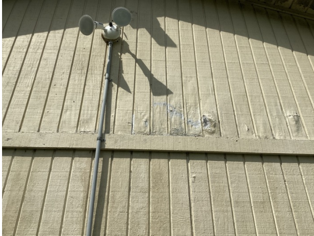
Wood rot at pool house
