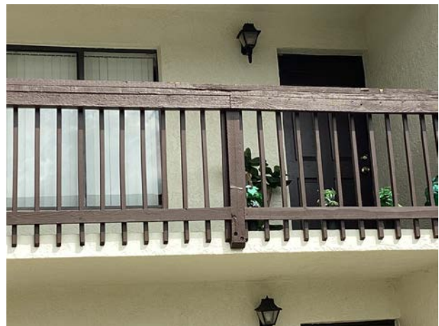
Damage at balcony railing
