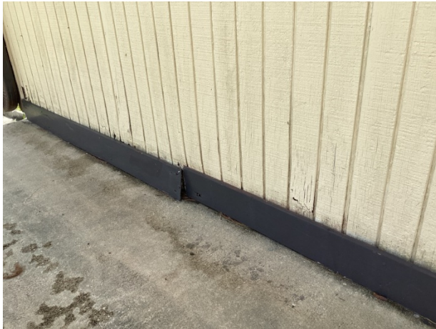
Wood rot at pool house
